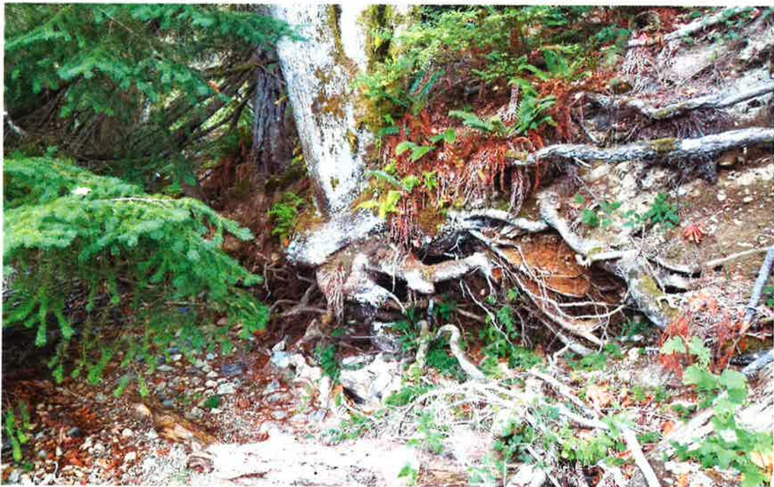
Photo 4: Conditions along the lakeshore adjacent to Slide 3 showing wave undercutting, road bank over steepening and erosion scour features. Facing northwest.
