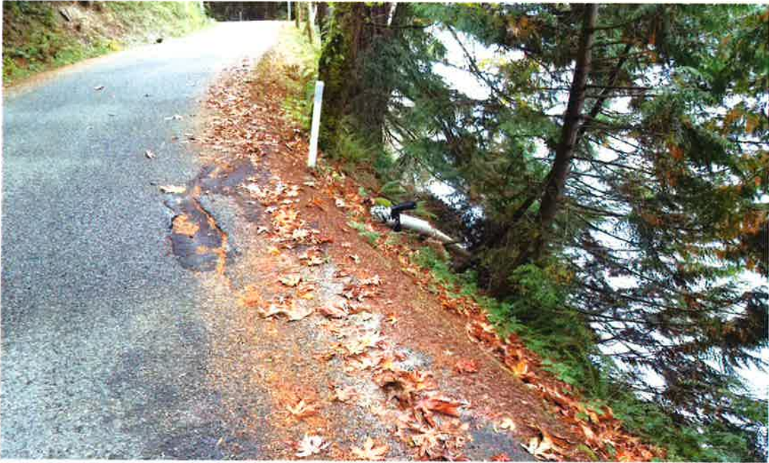
Photo 3: Slide 3 location showing existing conditions, including storm drain system in upper-center of picture. Facing east.
